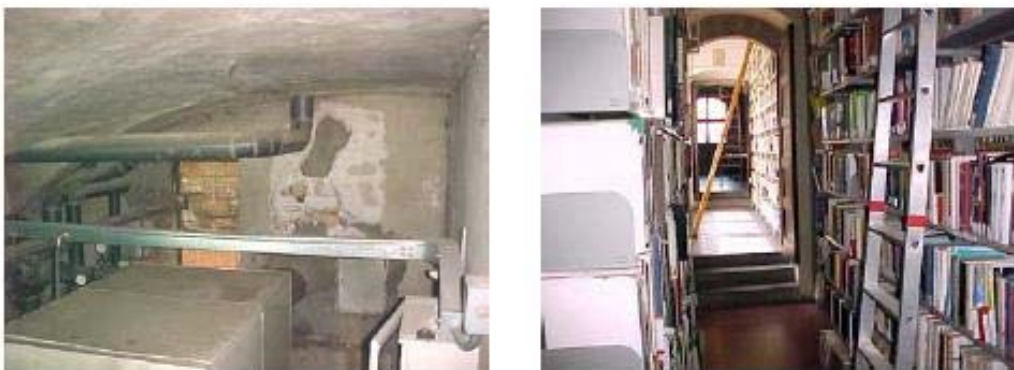
Figure 8: Heating plant and part of interior.
